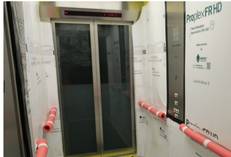
Little to No Maintenance
